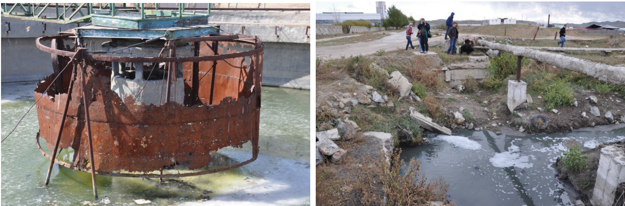
Figure 23 a.) Damaged clarifier of central WWTP b.) Discharge of untreated industrial wastewater from tannery towards Kharaa river
