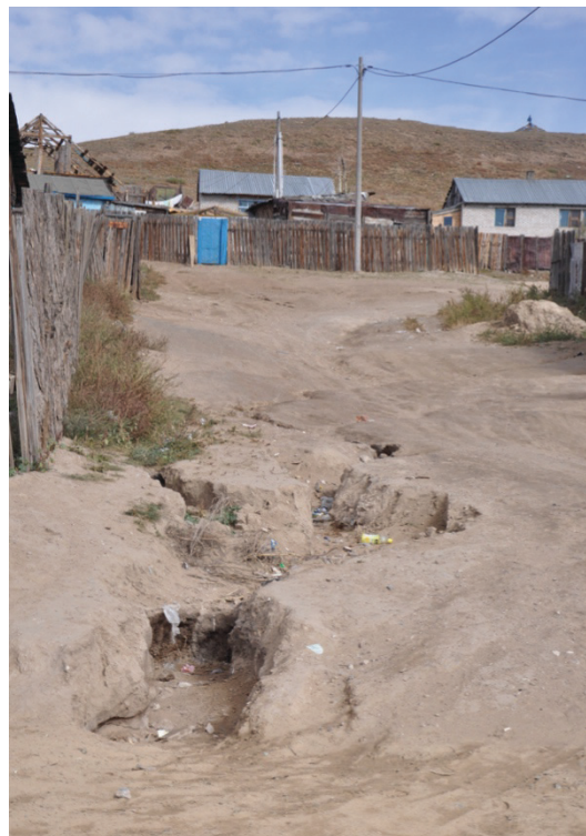
Figure 27: Lack of drainage & damaged road in bag7
