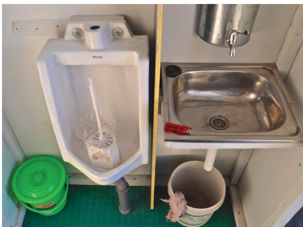
Figure 34: iPiT@ equipped with urinal (not used here) and wash basin
