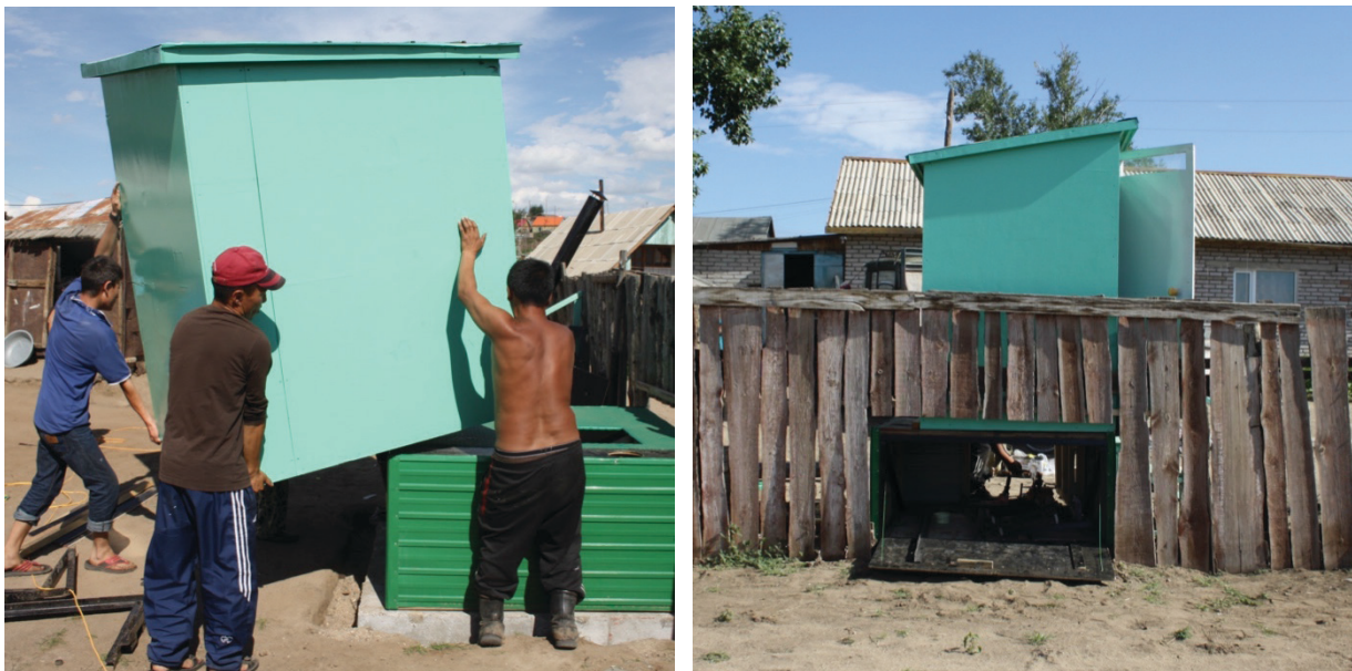
Figure 33: a.) Installation of toilet house b.) Finished installation of iPiT@ (photos: P.
